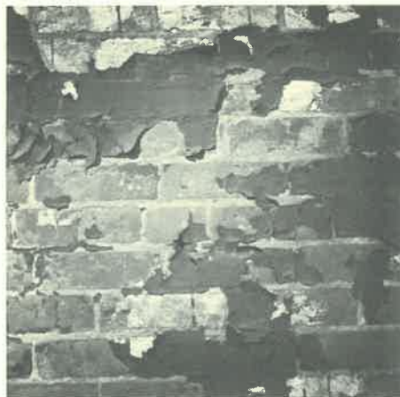
EXAMPLE OF PAINT ENCRUSTATION. TREATMENT: SCRAPE LOOSE PAINT AND REPAINT.
