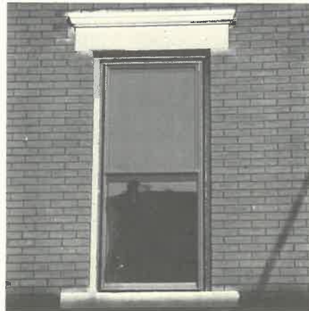
NEW DOUBLE HUNG WINDOW WITH DARK FRAME IS ACCEPTABLE. THIS IS A "ONE OVER ONE"
