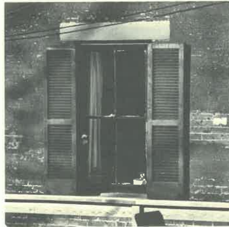
TYPICAL WINDOW IN PROSPECT HILL - WITH OPERABLE SHUTTERS. FASTENED TO CASING, NOT TO BUILDING. SIZED TO FULLY COVER WINDOW WHEN CLOSED.
