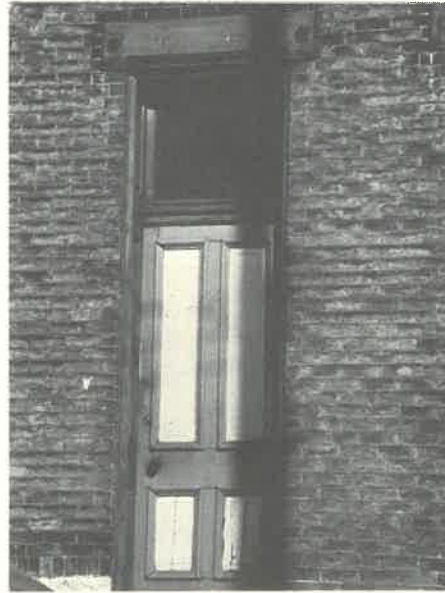
TYPICAL SIDE DOOR WITH PANELED WOOD DOOR, TRANSMOM WINDOW AND STONE LINTEL
